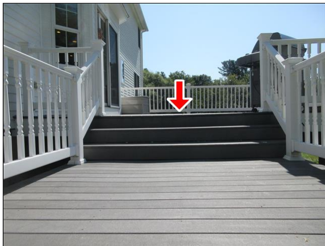
Upper deck bowed downwards
