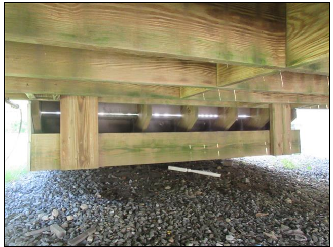
Lower deck and steps hung from a single joist at the upper deck
