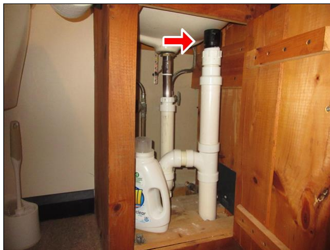
Internal vent at first floor bathroom sink
