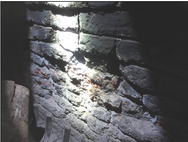
Deteriorated masonry at the back of the kitchen fireplace
