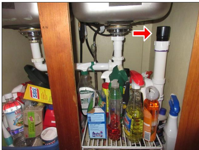
Internal vent at kitchen sink
