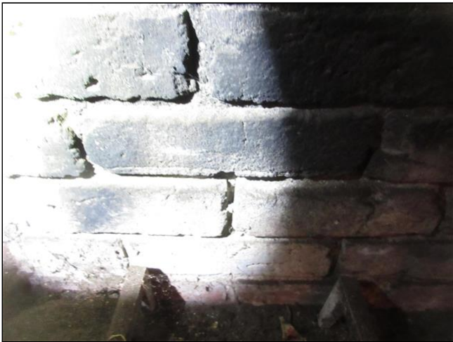
Deteriorated masonry at the back of the dining room fireplace
