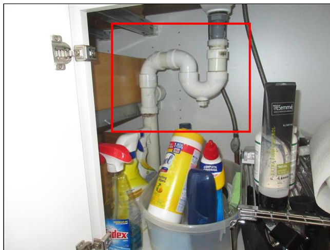
Unvented S trap at second floor bathroom sink drain
