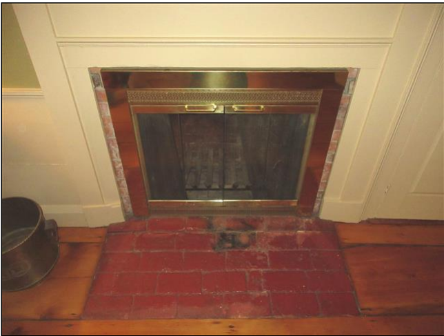
Wood too close to firebox
