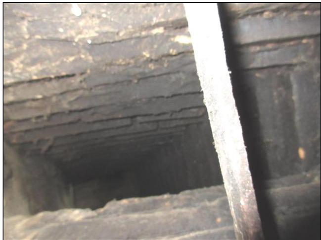
Unlined flue, no damper
