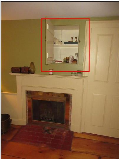
Wood in cabinet too close to the chimney
